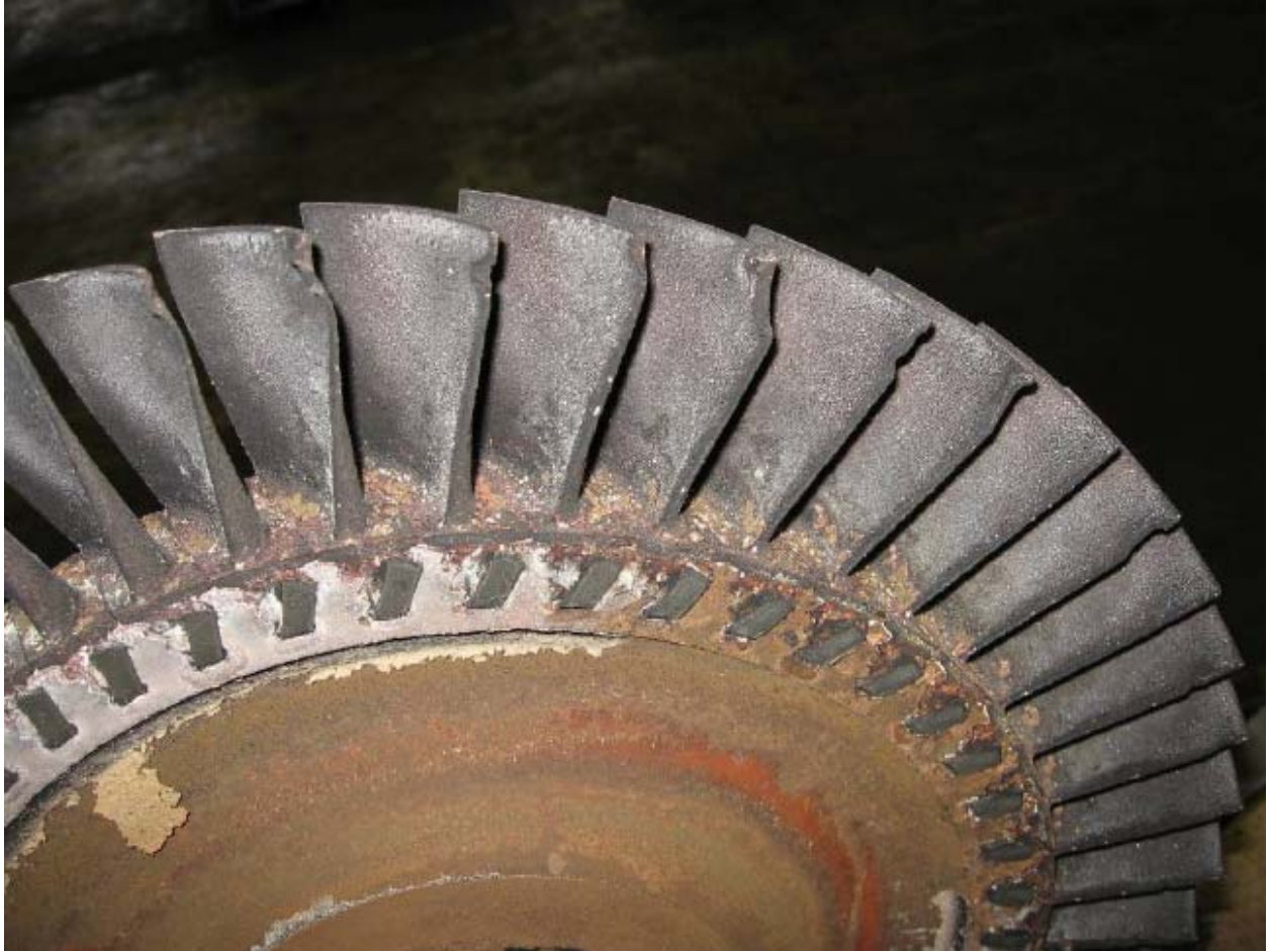
Figure 4: Foreign material damage to turbine wheel
