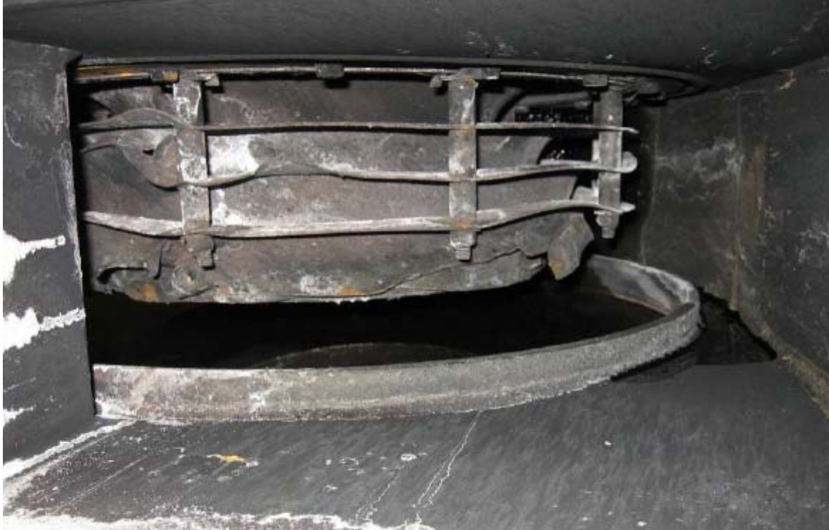
Figure 5: Warped exhaust diffuser
