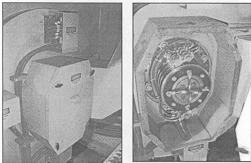
Figure 5 Main Generator Slip Ring Brush Compartment
