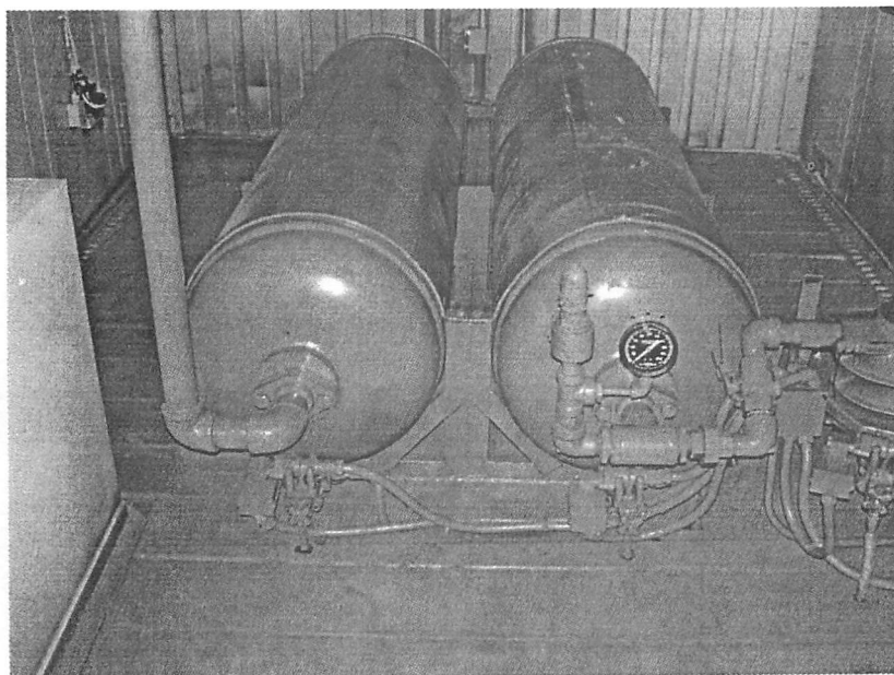
DBC main reservoir tanks
