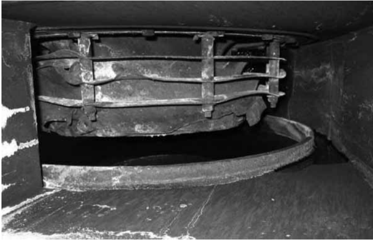
Figure 5: Warped exhaust diffuser
