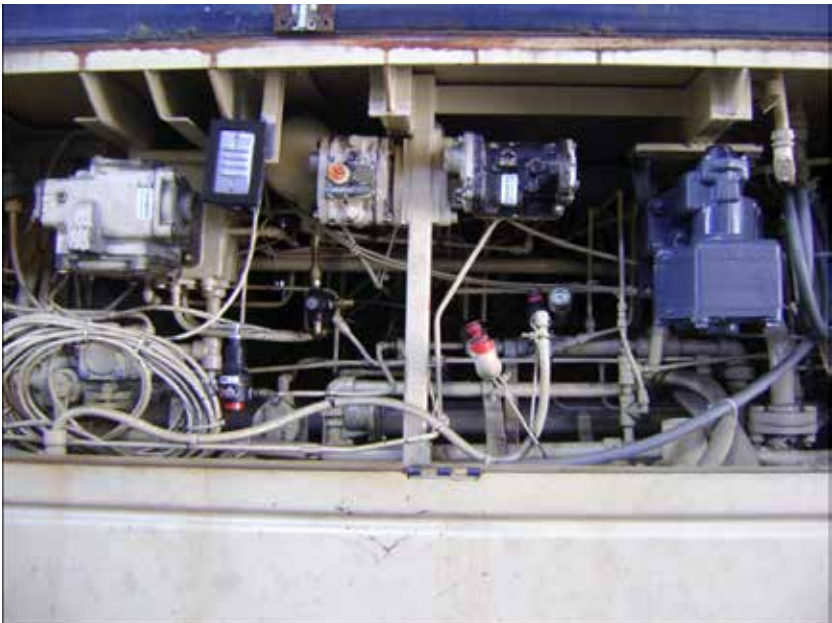
Figure 4. A 92 day maintenance interval brake system.
