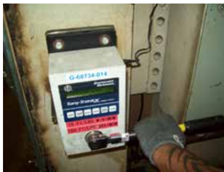
Figure 7: Improper Wrench Handling
