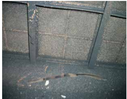
Figure 12: Finger Mark in Soot before Cleaning
