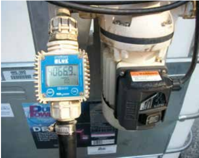
Figure 23: Pump System on Urea Tote
