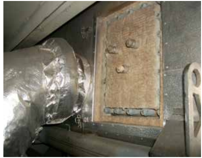
Figure 10: Inspection and Cleaning Access to DPF
