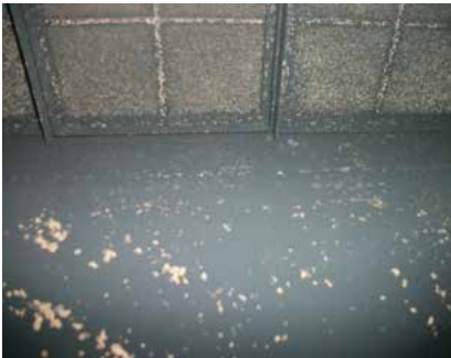
Figure 11: Interior of DPF before Cleaning
