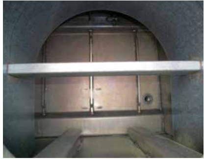
Figure 14: Interior of Exhaust after 5,083 Hours
