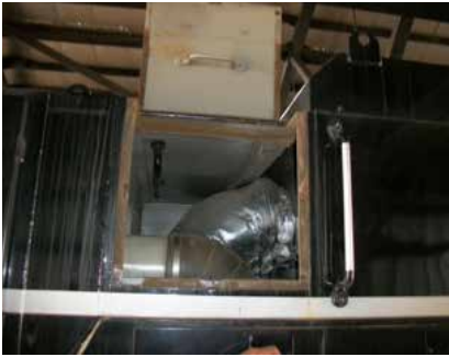
Figure 9: Access for DPF Cleaning and Inspection
