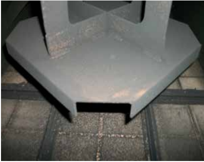
Figure 13: Exhaust Diffuser in DPF before Cleaning
