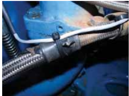
Figure 11 – Cable tying improvements
