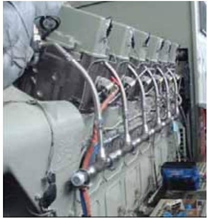
Gas manifold on a GE engine
