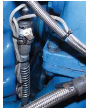
Figure 7 – Water pressure transducers, slack cable
