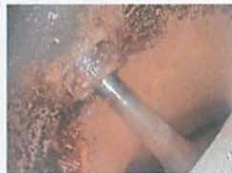
Intake Port Badly corroded
