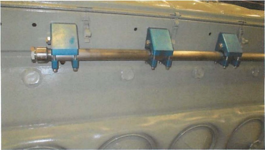
Figure 6. Natural Gas Manifold on side of 645E engine.
