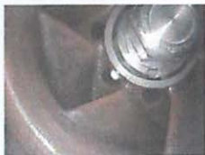
Rotor Inspection Some Corrosion, but Still Operable
