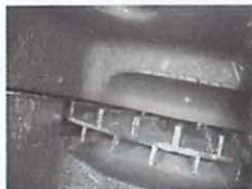
Pump Heat Sink Made visible with video borescope
