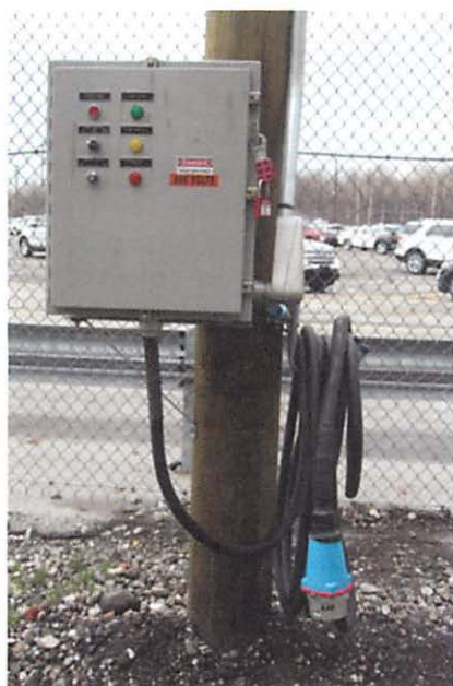
Figure 5: Conventional Plug In Station
