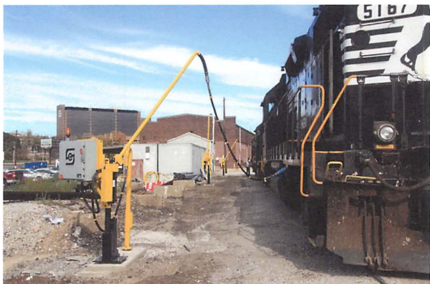
Figure 7: Snyder Equipment Co. electric Plug-in Station at North Kansas City Yard
