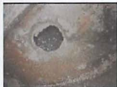
Surface Corrosion Should Have Borescoped This Area Long Ago
