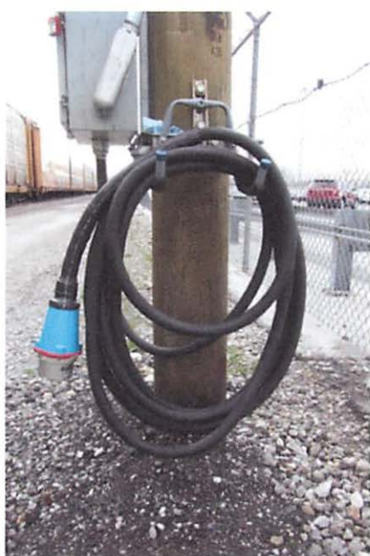
Figure 6: Shore Connection Cable
