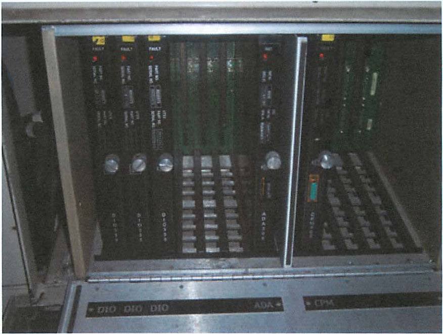
Figure 1. Locomotive Computer Chassis with 3 DIO Modules
