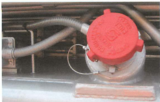
Vent hose correctly applied
