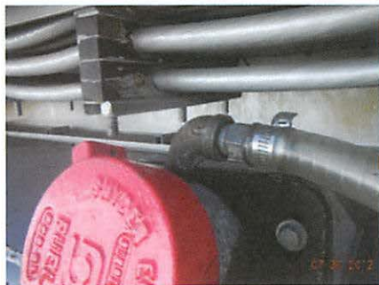
Incorrect hose and fittings
