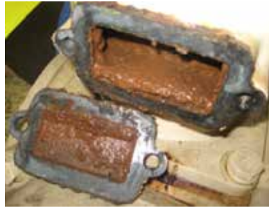
Rust/ Sludge in air compressor
