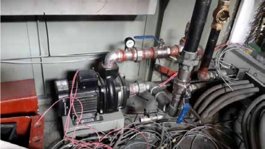
Figure 17: AC cooling pump in ATS system. Cooling pumps are required to move coolant from inverters to radiator. (Used with permission)
