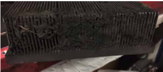
Figure 20: Dirt and debris accumulated on inverter cooling fins.
