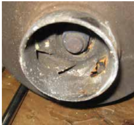
Corrosion on a water pump
