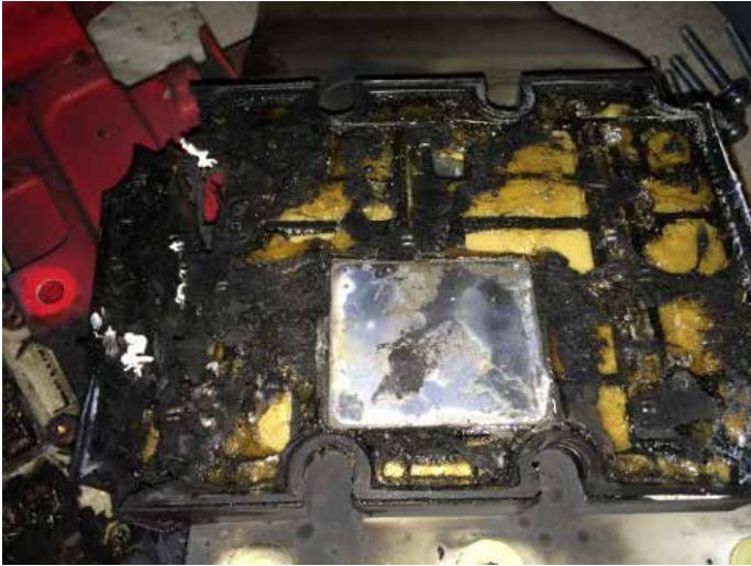
Figure 18: Innards of an inverter after cooling failure.
