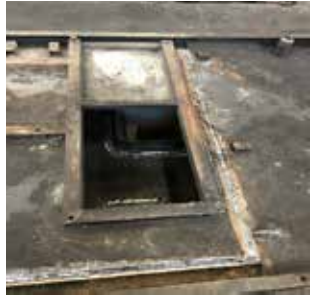
Rear Platform (Under the Rad Cab)
