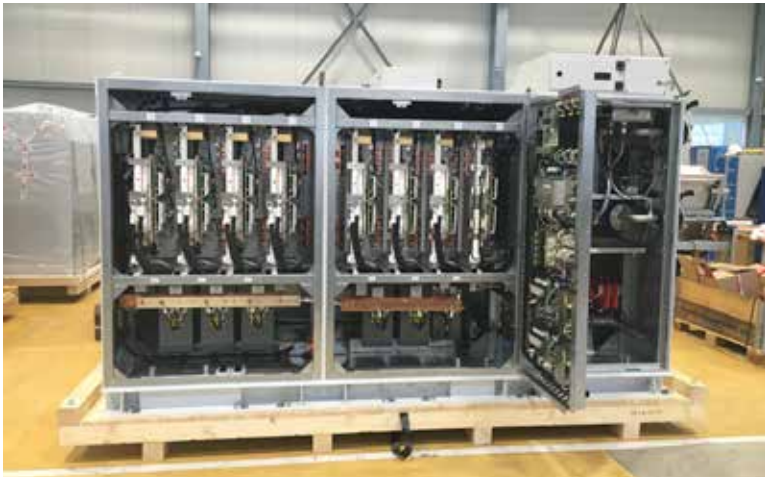
Figure 1: An example of a GTO to IGBT upgrade. Note the 3-level topology with liquid cooling system on the right. (Go to https://youtu.be/w2IOjZnCcZY for Youtube presentation. Used with permission.)
