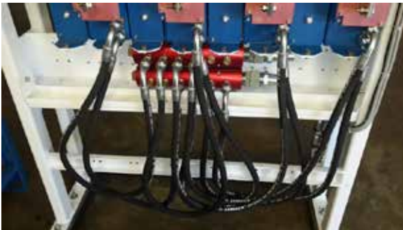
Figure 16: Cooling pipe and manifold arrangement on ATS liquid cooled inverter system. (Used with permission)
