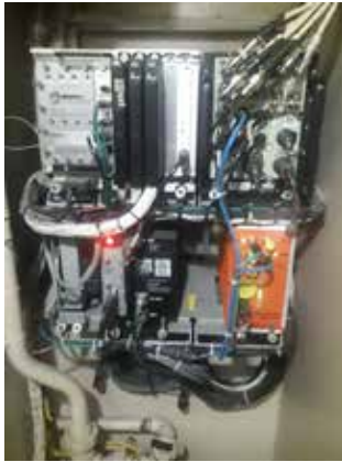
Figure 6: Onboard equipment that is usually installed in the nose of the locomotive consists of the Train Management Computer (TMS), Event Recorder, and Crash-Hardened Memory Module (CHMM).
