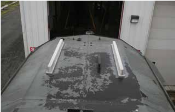
Figure 7: Roof of locomotive cab showing the new installation of antennae arrays to support the PTC installation, and to allow communication between the locomotive and wayside equipment.
