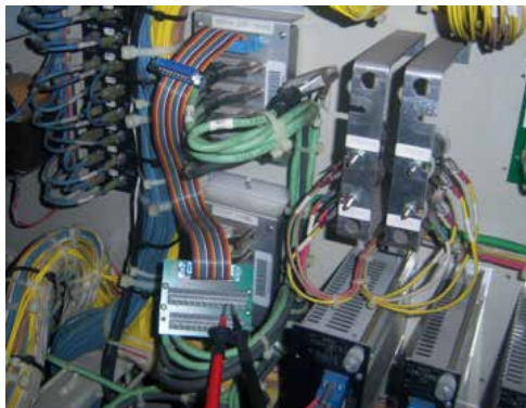
Figure 13. Serial Distribution Panel
