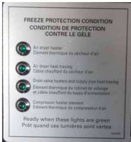
Figure 6 – Freeze protection monitoring Display panel
