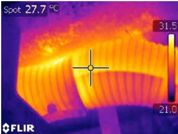
Figure 5 – Freeze protection – Thermography of the air conduit heat tracing
