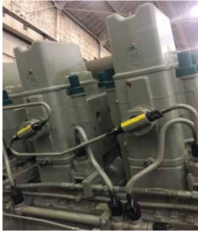
The piping is inviting as a handhold.
