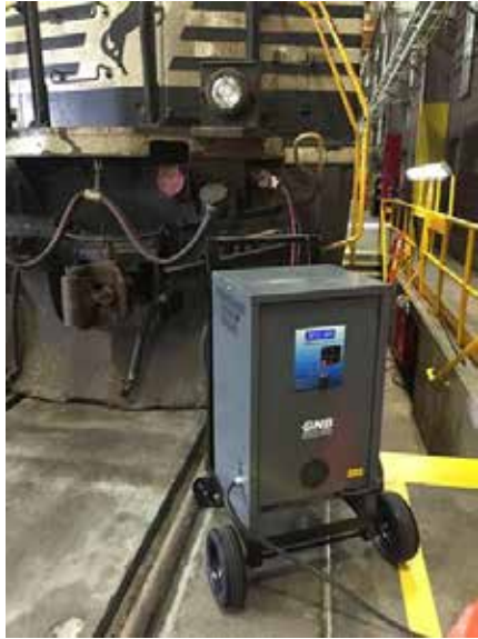
Figure 11. Shop Battery Charging
