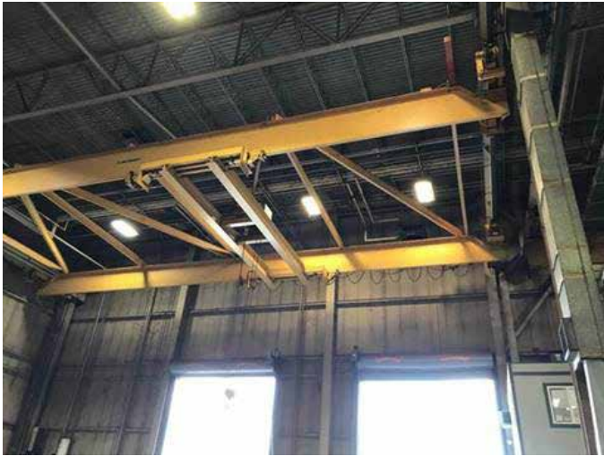
Figure 2. Overhead Bridge Crane
