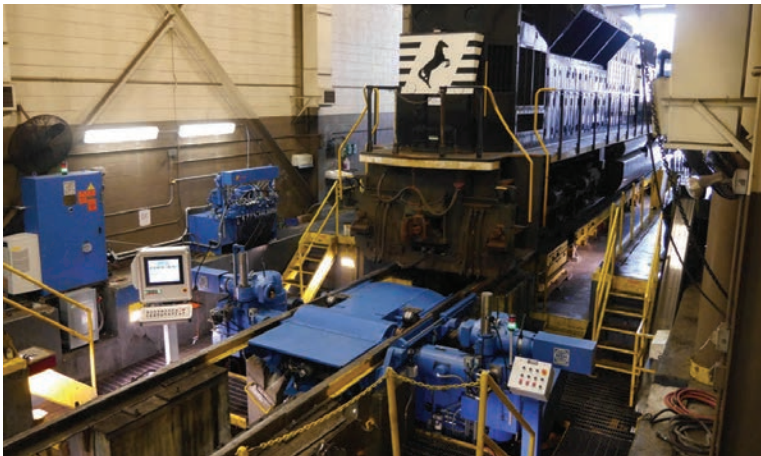
An underfloor wheel truing machine installation
