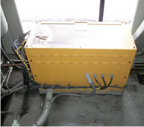
Figure 9: DEF Dosing Cabinet
