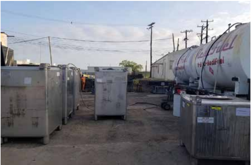
Figure 2. Fuel Storage Tanks
