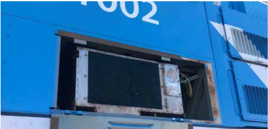
Picture 7: Progress Rail (EMD) Sub-Base HVAC Type
