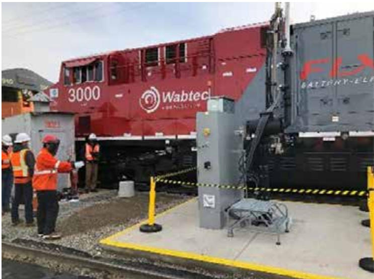
Figure 5 Image of BEL While Charging at the BNSF Stockton Mormon Yard
