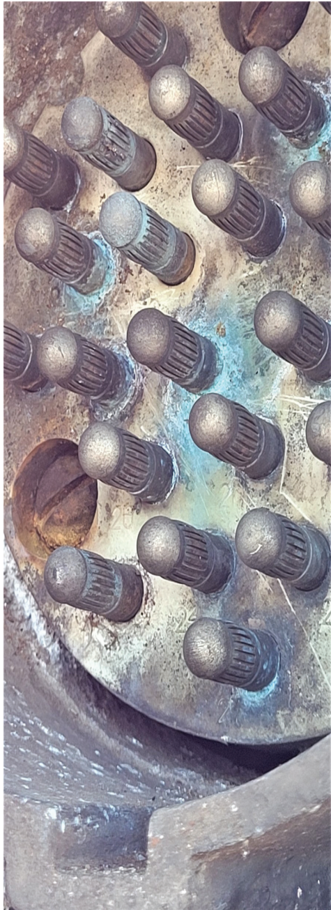
Figure 12: MU Receptacle issue: Pin Damages
