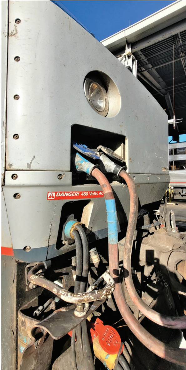
Figure 2: 27 Point Trainline Communication Cable (Blue)
