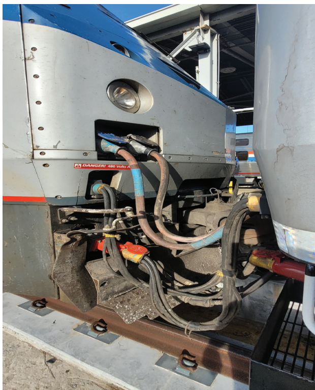
Figure 7: MU Jumper Cable installed between Locomotives
