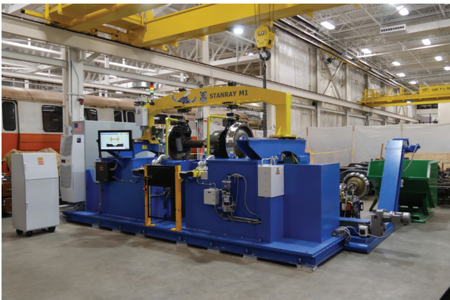
An above-floor wheel truing machine installation
