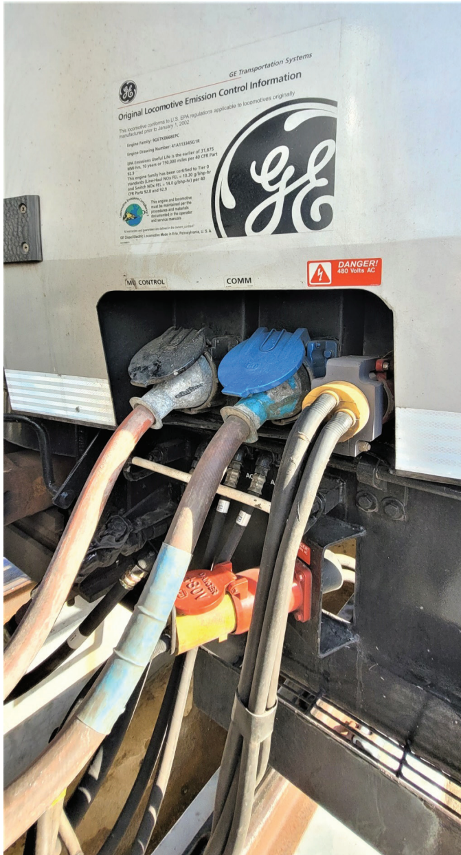
Figure 3: 27 Point Trainline MU Cable (Black)
