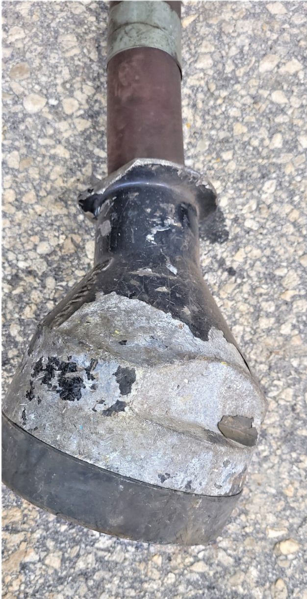
Figure 14: MU Jumper Cable Issue: Plug damages
