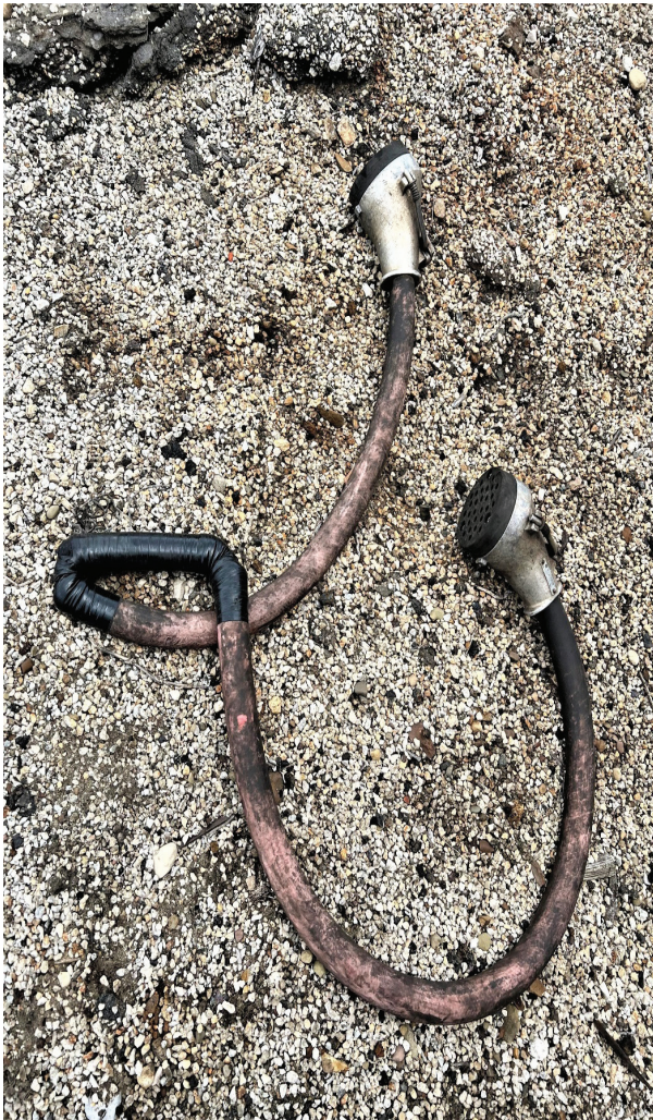
Figure 13: MU Jumper Cable: Insulation Integrity Damages
