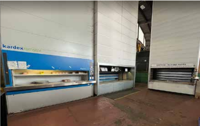
Large Material Carousels, CSX Nashville, TN
