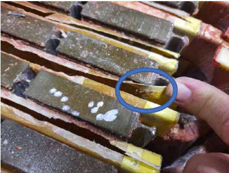
Figure 8: Insulation defect identified with visual inspections.
