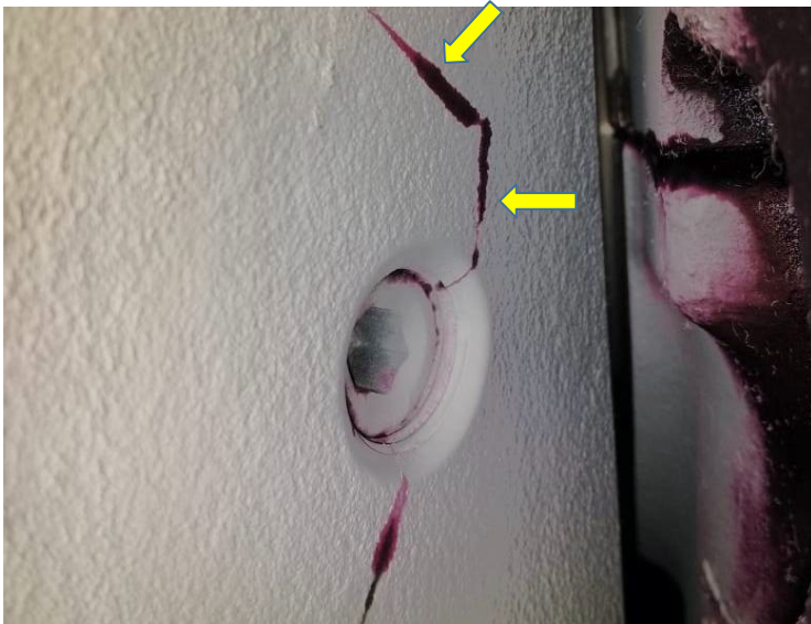
Figure 9 - Cracks are too long
