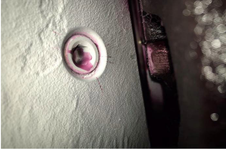
Figure 5 - Initial and small cracks
