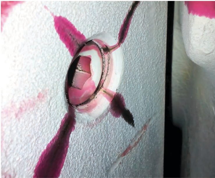
Figure 12 - Four legs crack
