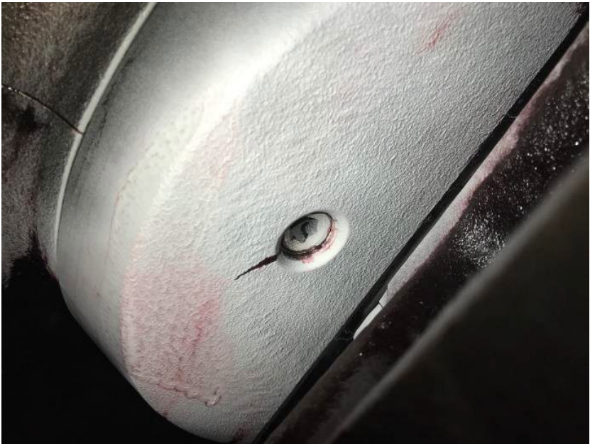
Figure 7 - Advanced single crack leg
