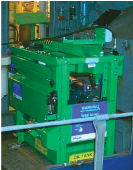
Fig 1 Auxiliary Power Units
