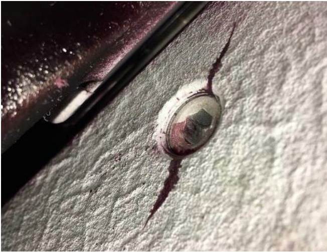
Figure 8 - Two crack legs
