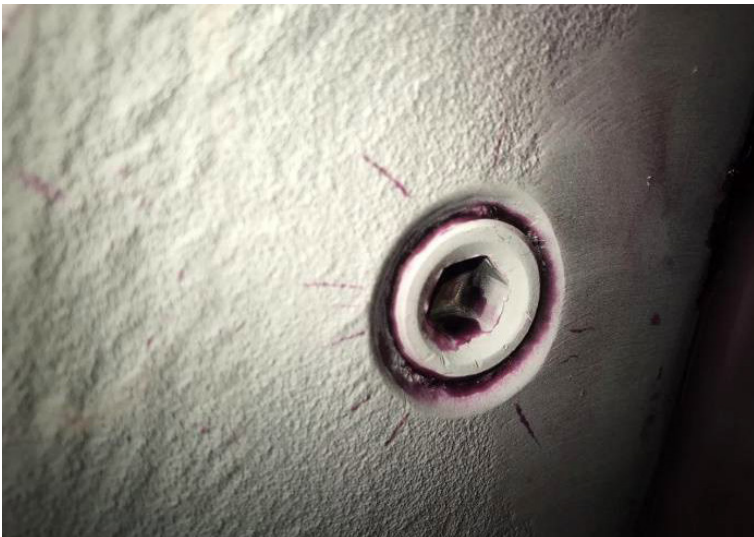
Figure 6 - Cracks around the hole
