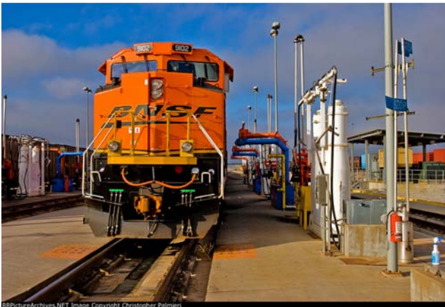
FIGURE #1 Locomotive on Fueling Pad (BNSF Railway in Lincoln, NE image courtesy of Chris Palmieri)
